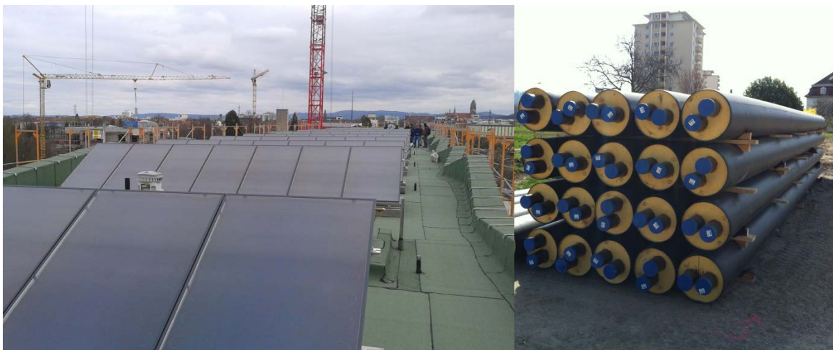
Figure 15: View on collector array of the largest plant in the urban quarter "Gutleutmatten" as well as the piping-system of the heat network. (Source: Fraunhofer ISE, badenovaWÄRMEPLUS GmbH & Co. KG)
