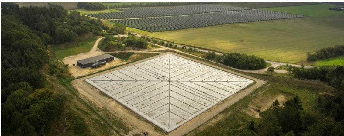
Figure 3: Pit heat storage in Dronninglund with the solar collector field seen in the back (Source: Dronninglund Fjernvarme A.m.b.A)
